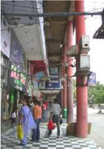
AC UNITS (CONDENSER AND COMPRESSOR) HAVE BEEN PROVIDED IN COMPULSORY PUBLIC CORRIDOR
