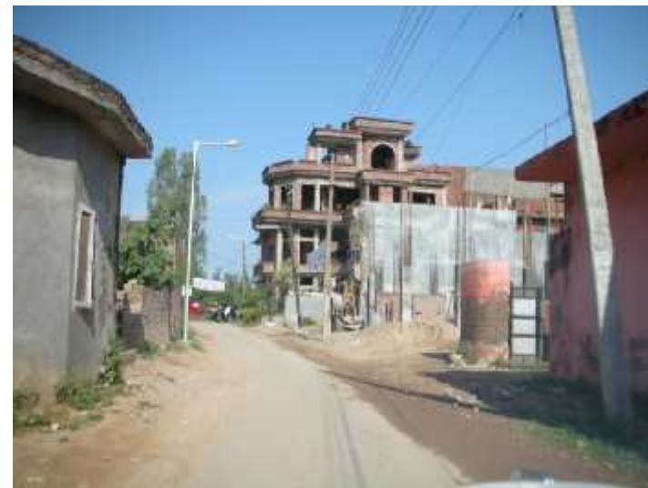
NEW CONSTRUCTION ACTIVITY BEYOND MAXIMUM PERMISSIBLE HEIGHT IN VILLAGE SARANGPUR
