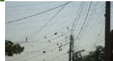
OVERHEAD WIRES –ILLEGAL CONNECTIONS
