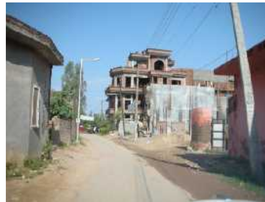
NEW CONSTRUCTION ACTIVITY BEYOND THE MAXIMUM PERMISSIBLE HEIGHT VILLAGE SARANGPUR
