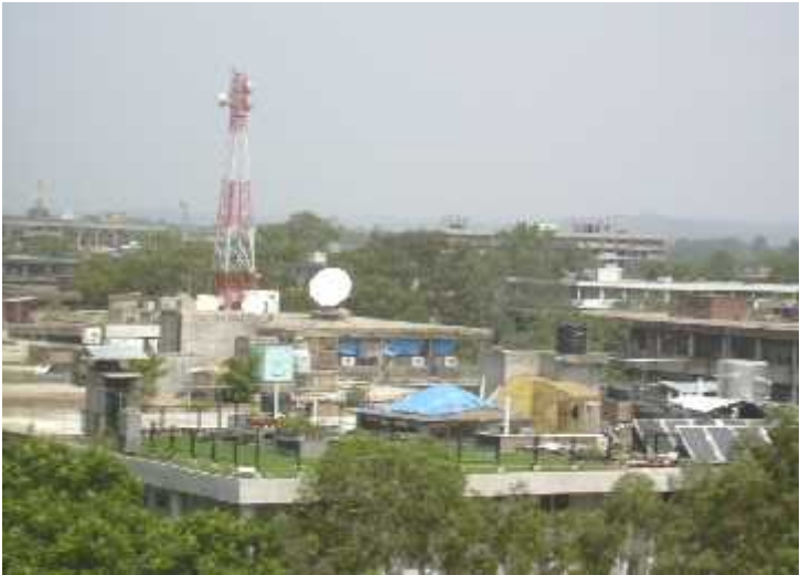
UNAUTHORIZED CONSTRUCTIONS ON TERRACE, SUCH AS TEMPORARY STORES, DISH ANTENNA, CABLE TOWERS ETC.
