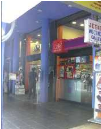
UNAUTHORISED PAINTING OF FACADE & COLUMNS
