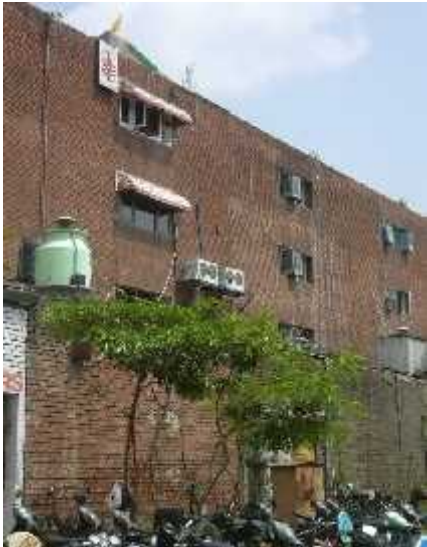
OPENING OF ILLEGAL SHOPS ON THE REAR OF BRICK FACED SCOS TOWARDS PARKING SIDE.
