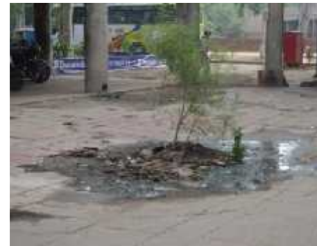
BROKEN PLAZA FLOORS WITH UNEVEN SLOPE DIRECTIONS CAUSING STAGNATION OF WATER
