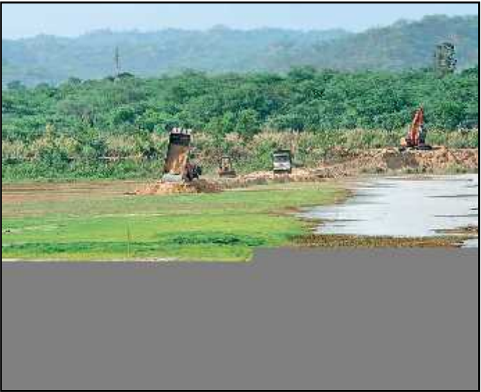
PROBLEM OF SILTATION IN THE LAKE
