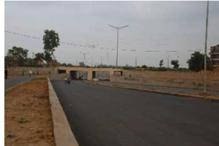
RUB with NMV facilities – first of its kind provided in Chandigarh along Route No. 2
