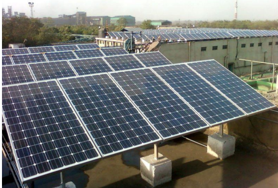
100 KW SPV Power Plant Installed at SEML, Siltara, Raipur
