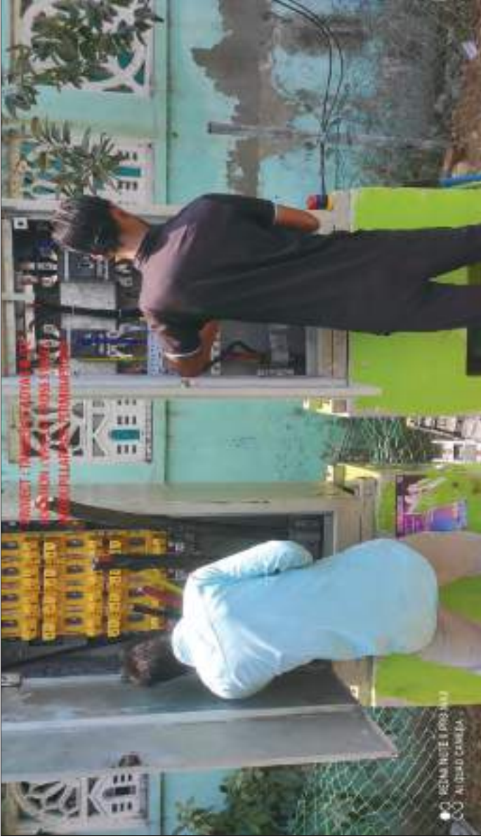
Cable Termination at Pillar Box – Adyar & ITC Division
