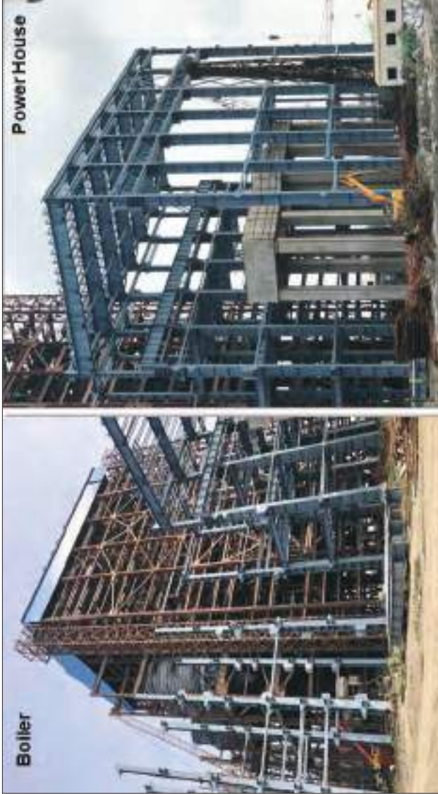
Ennore SEZ Thermal Power Project
